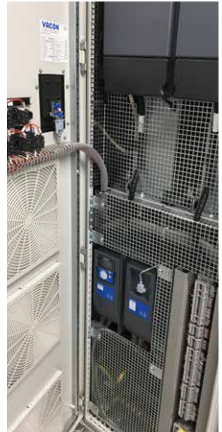
Detail of the electrical panel made by Casagrande Elettrocostruzioni housing Danfoss Drives VACON® NXP
