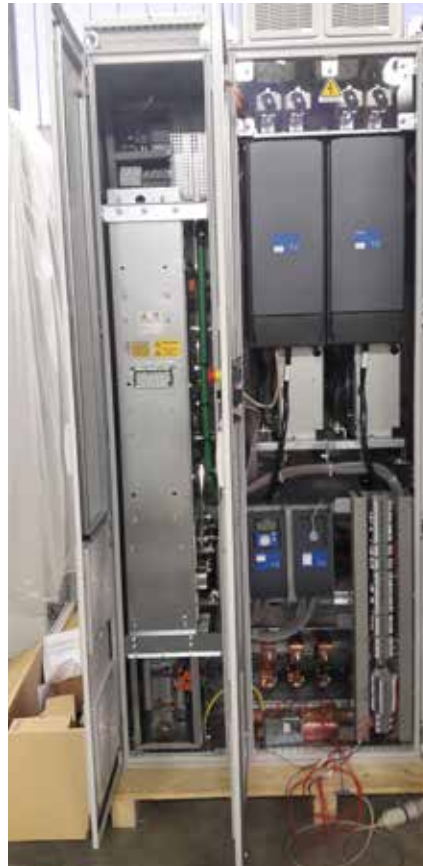
Electrical panel for the waste plant in Edinburgh during the final testing at the Casagrande Elettrocostruzioni factory in Verona
