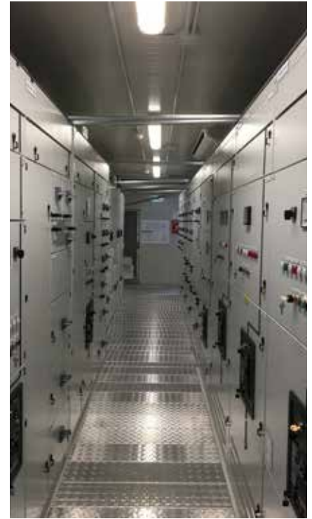
Inside view of a container made by Casagrande Elettrocostruzioni for the Edinburgh Energy from Waste plant
