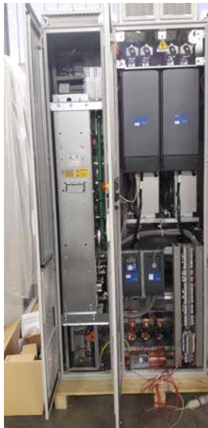
Electrical panel for the waste plant in Edinburgh during the final testing at the Casagrande Elettrocostruzioni factory in Verona
