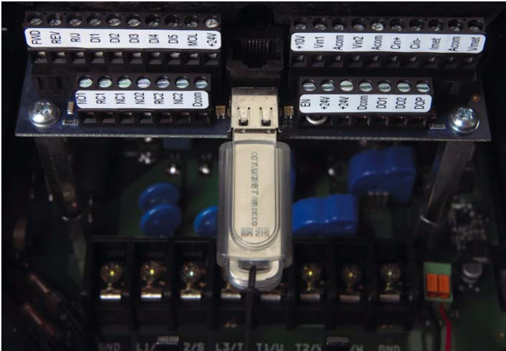
Figure 9: Vacon 500x Control Terminals
