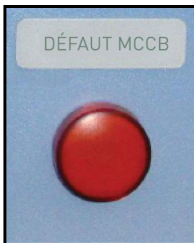
Figure 29. Voyant LED MCCB FAULT
