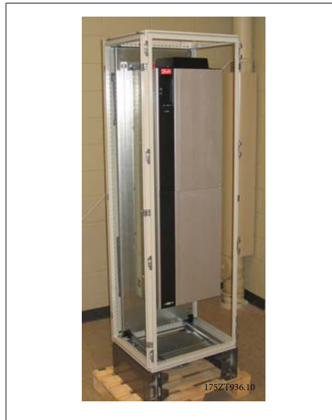
3.36: Adjustable frequency drive installed in cabinet
