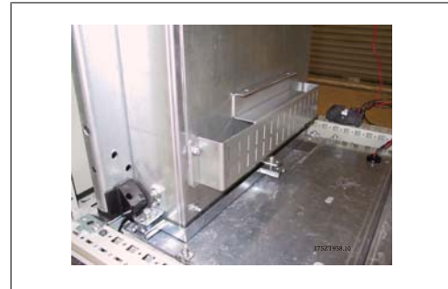
Illustration 3.59: Gaine inférieure installée
