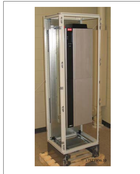
3.36: Adjustable frequency drive installed in cabinet
