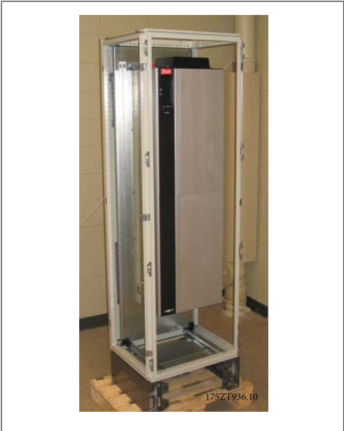
Illustration 3.36: Frequency converter installed in cabinet
