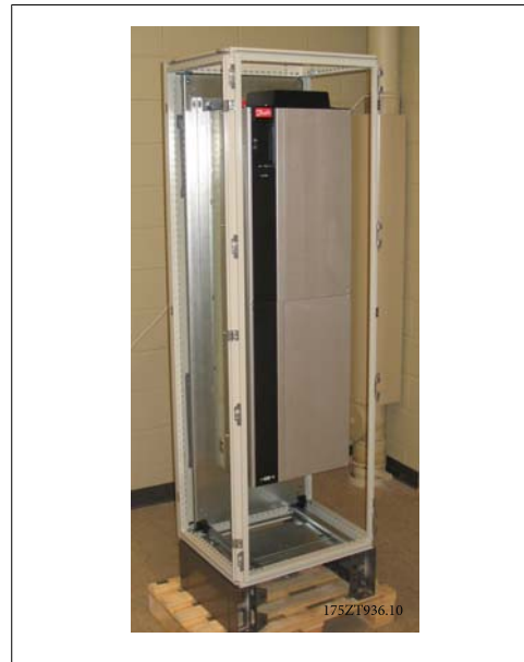
3.36: Adjustable frequency drive installed in cabinet
