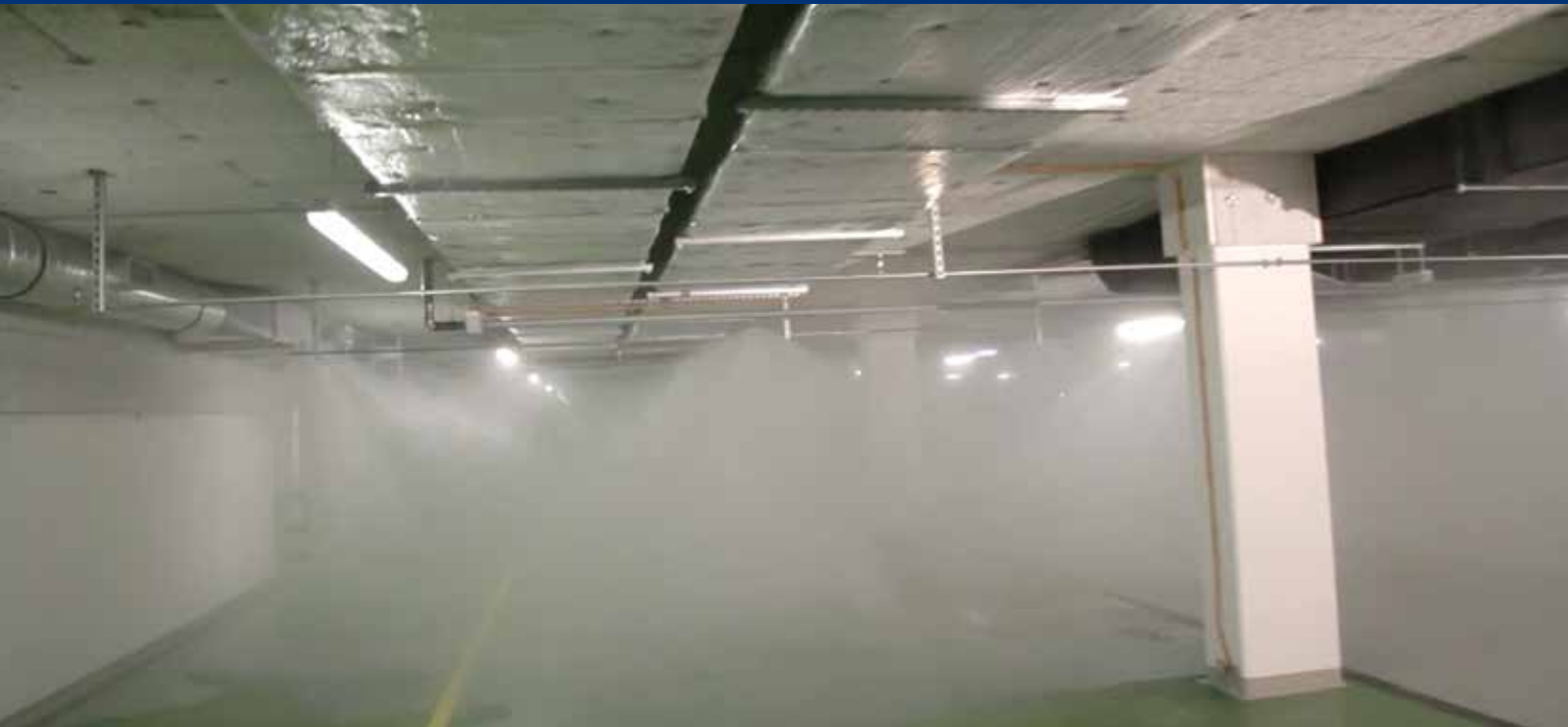
Budapest Air Traffic Control Centre - picture from test in underground car park, fully protected with Danfoss Semco SEM-SAFE® high-pressure water mist system
