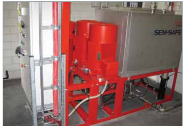
Compact Danfoss Semco pump unit installed at Equinix AM3
